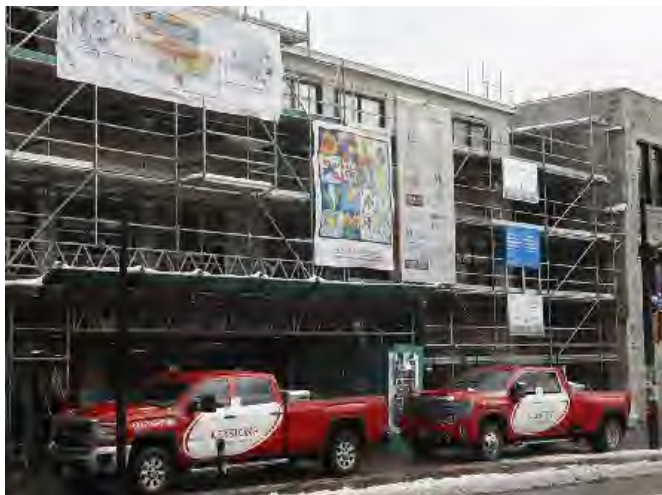
Bronson Centre Theatre is open for business during renovations. PHOTO BY TONY CALDWELL /POSTMEDIA
